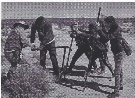
Teamwork! Lancaster High School students join their teacher, Glen Baumbach in removing old fencing posts.
